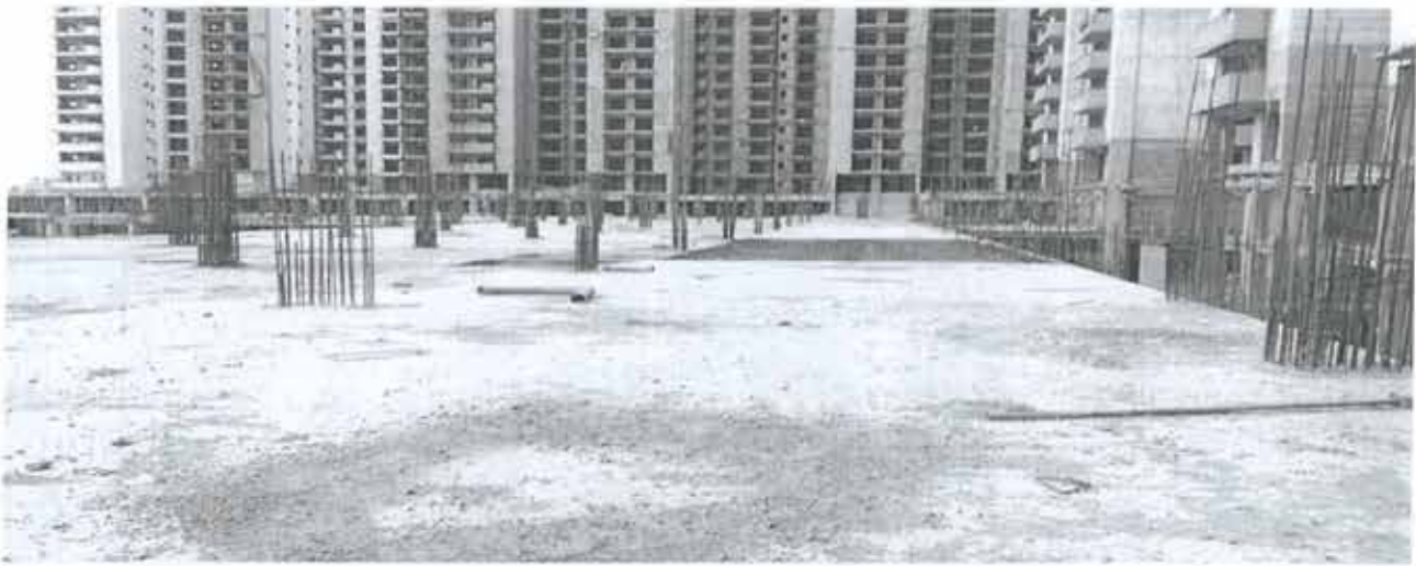
T-4 TO T-6 REAR SIDE NON TOWER TOWER CENTRAL AREA COLUMN & SLAB CASTING
