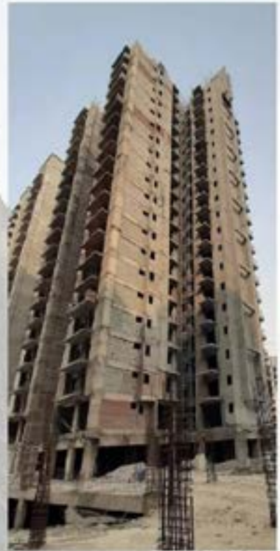
TOWER T-6 SIDE
