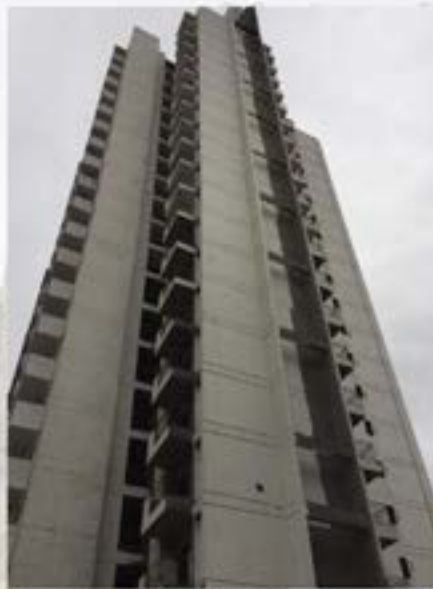
TOWER T-4 SIDE
