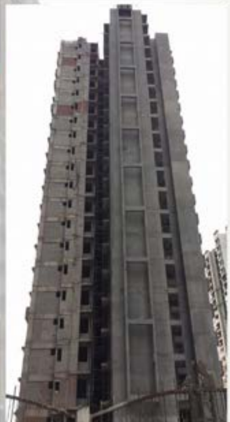
TOWER T-6 SIDE
