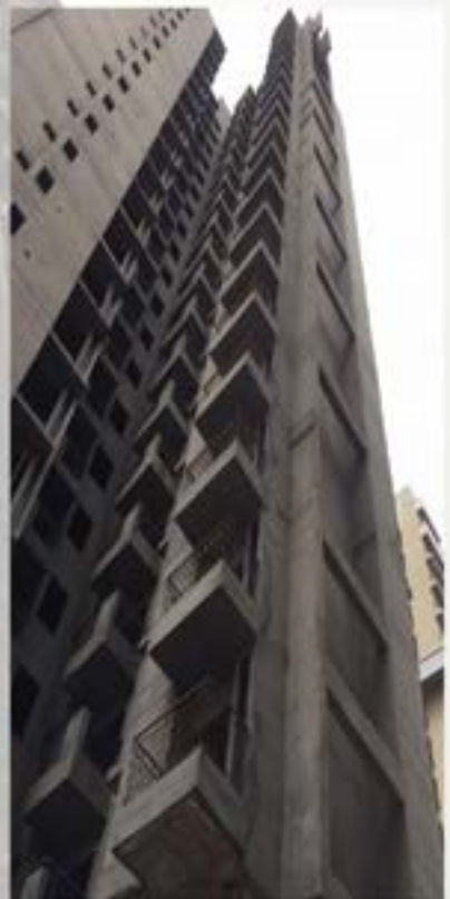
TOWER T-9 SIDE
